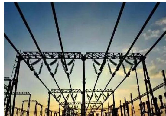
Phnom Penh-Bavi power supply Project activated
